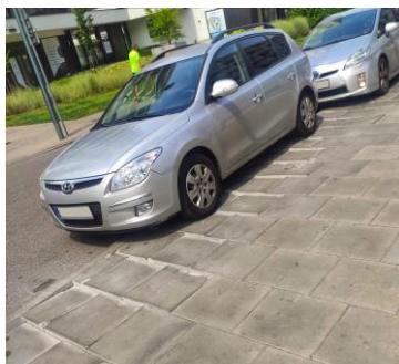
Fig. 6. Destruction of the pavement on Komputerowa Street.
