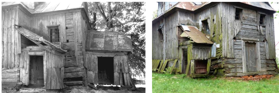
Fig. 5. Mięgisz Stary, progressive degradation of the church's construction structure: state in 1989 (left) and existing state in 2015. Source: photo by author
