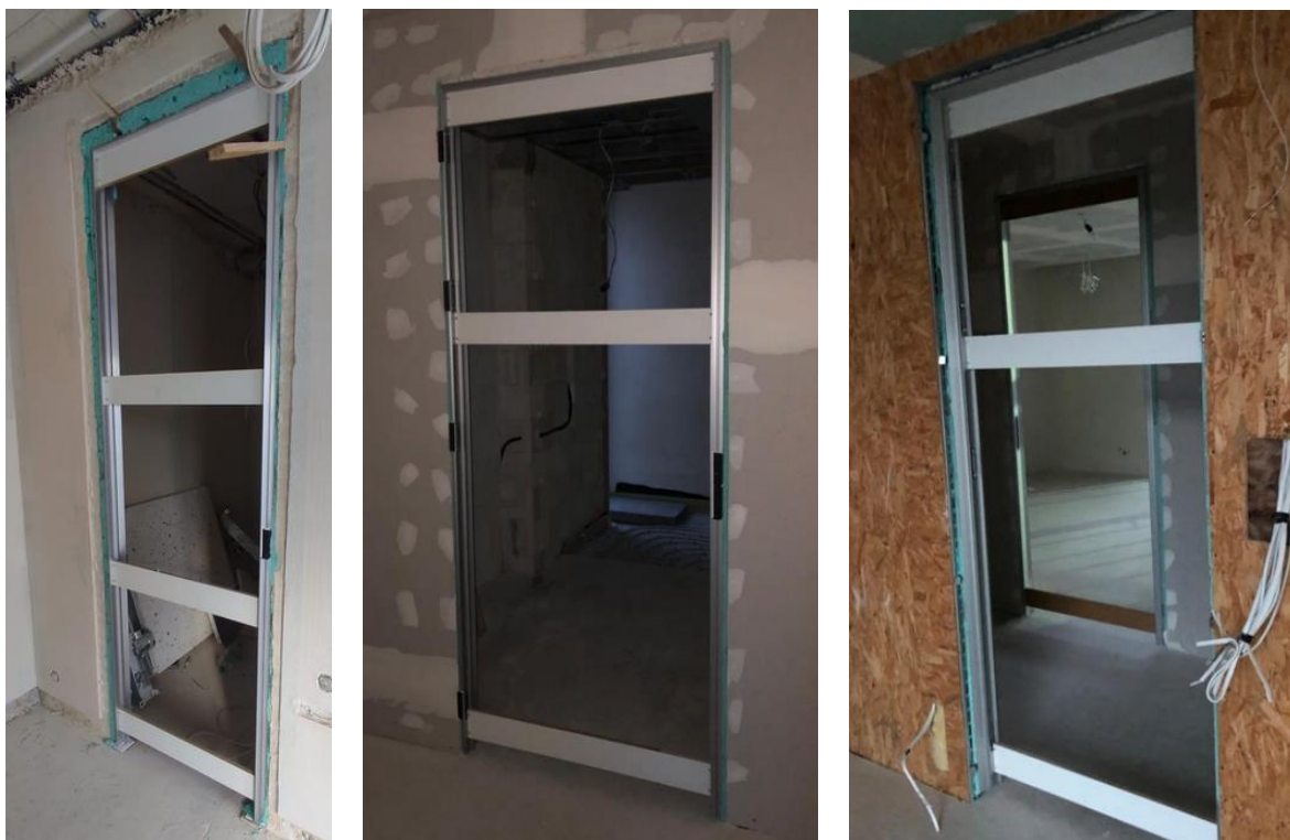
Figure 3. Photos showing the assembly of the door frames in the walls finished with drywall boards - gypsum-cardboard and wood-based boards. different finishes Source: Photos from the archives of the Zeromur company.
