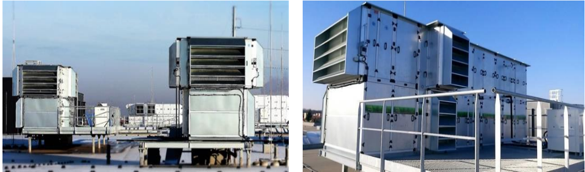
Fig. 10. View of an efficient control station Warszawa and Mielec. Source: the authors.
