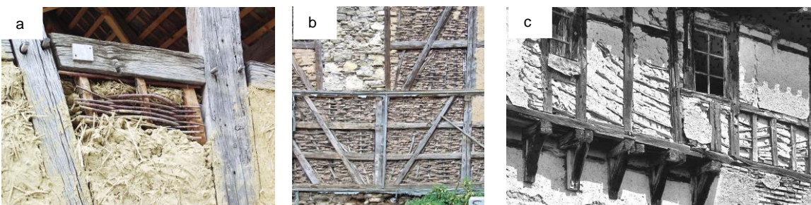
Fig. 4. Examples of filling the frame space fields with braids made of branches, wicker or wooden patches and plastering the internal and external surfaces with clay.
