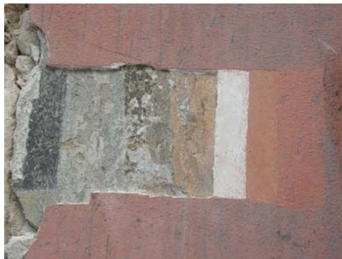
Fig. 4. Sounding of painting layers of the façade in 28, Market Square. The red color appears only in the 20 th century. Source: photo by author
