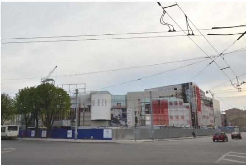
Fig. 3. Former factory JSC "Gas Equipment". Construction of the new shopping centre Forum Lviv. Source: photo Y. Senkovska
