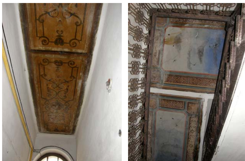
Fig. 18. Early Historicism murals of the house in 39 Rynok Sq.: in the pathway to the courtyard (tempera painting on the wooden board) and on the upper store of the staircase (open sky with swallows). Nowadays the last one is destroyed during the reconstruction of the house for hotel. Source: photo by author
