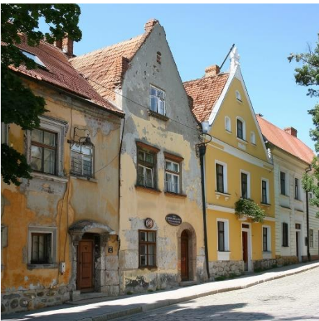
Fig. 26. Image generation output from Midjourney V6 with the prompt "Suwalki", yet again depicting a mismanaged, run down section of an old street. Visible degradation of facades, lack of general maintenance is visible in the generated content. Source: by author
