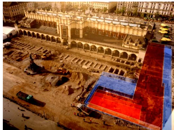
Fig. 2. Kraków. Market Square. Archaeological works and construction of the underground museum. Source: Historical Museum of Kraków, exhibition poster., photo: T.B-B. 2012.
