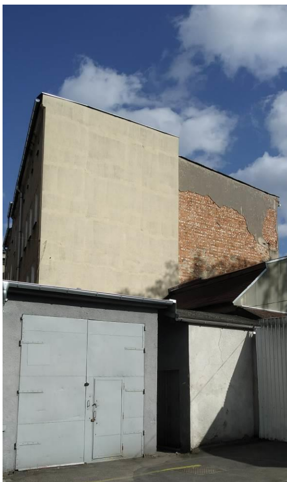
Fig. 7. Peeling plaster revealing the brick structure of the building. Source: Jarosław Piesik
