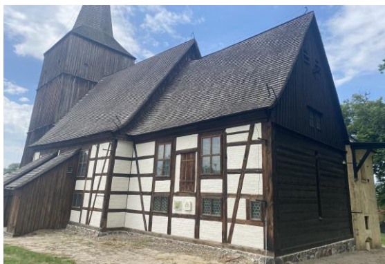
Fig. 3. Kłępsk, church of the Nativity of the Blessed Virgin Mary – the oldest west wall from 1367-1377 (mixed structure system - group 2). Source: autor's photo.
