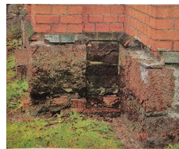
Fig. 6. Soggy foundation wall. Source: Photo collections of Andrzej Rybarczyk and Mirosław Hamberg
