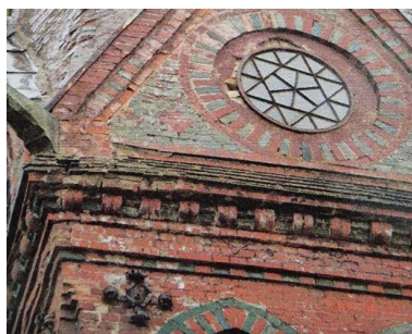
Fig. 5. Tower cornice with visible cracks. Source: Photo collections of Andrzej Rybarczyk and Mirosław Hamberg
