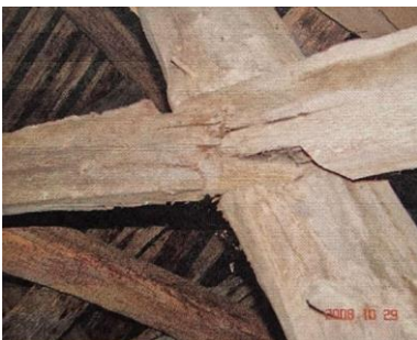
Fig. 7. Destroyed roof truss connections. Source: Photo collections of Andrzej Rybarczyk and Mirosław Hamberg
