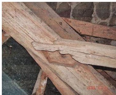
Fig. 8. Destroyed connections of the braces to the rafters. Source: Photo collections of Andrzej Rybarczyk and Mirosław Hamberg
