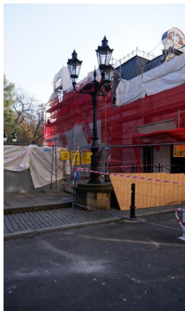
Fig. 5. Renovation of the Machinery House at the Juliusz Słowacki Theater in Krakow, October 2021. Source: photo by the author
