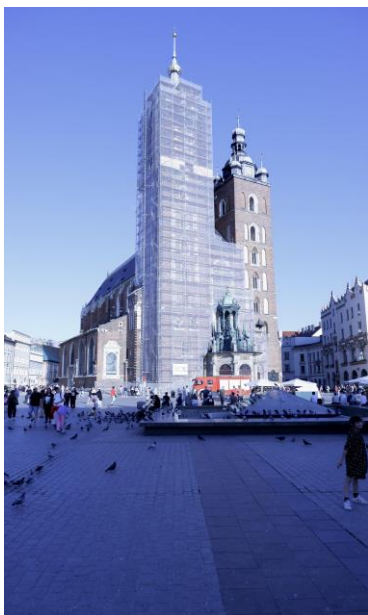
Fig. 3. Conservation of the tower of St. Mary's Basilica in Krakow, April 2024. Source: photo by the author
