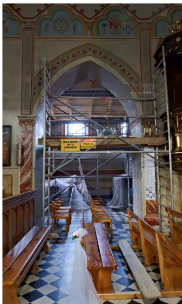
Fig. 4. Conservation of the interior of St. Michael the Archangel Church in Ujanowice, October 2020. Source: photo by the author
