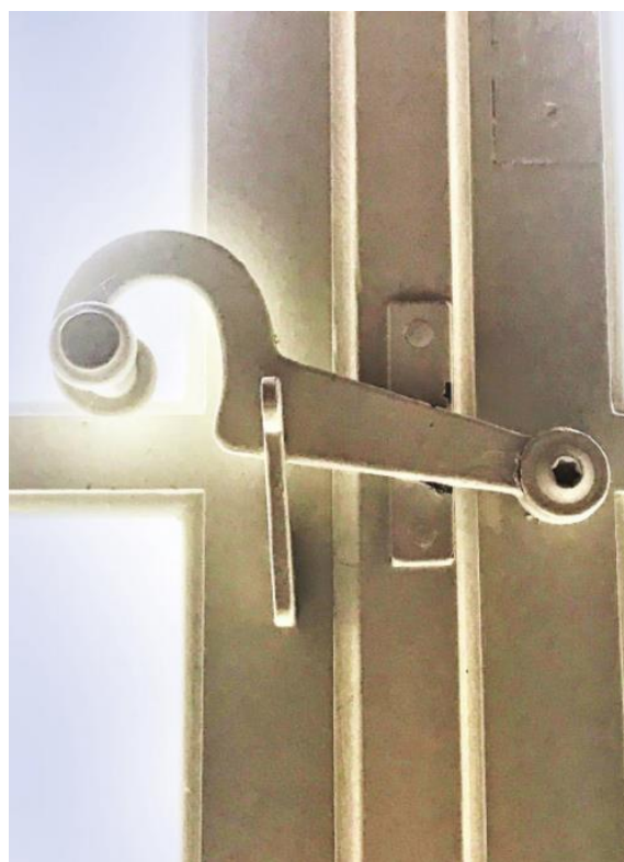
Fig. 7. Krakow, ul. Poselska 7. The photo shows the original window latch after renovation. Source: author.
