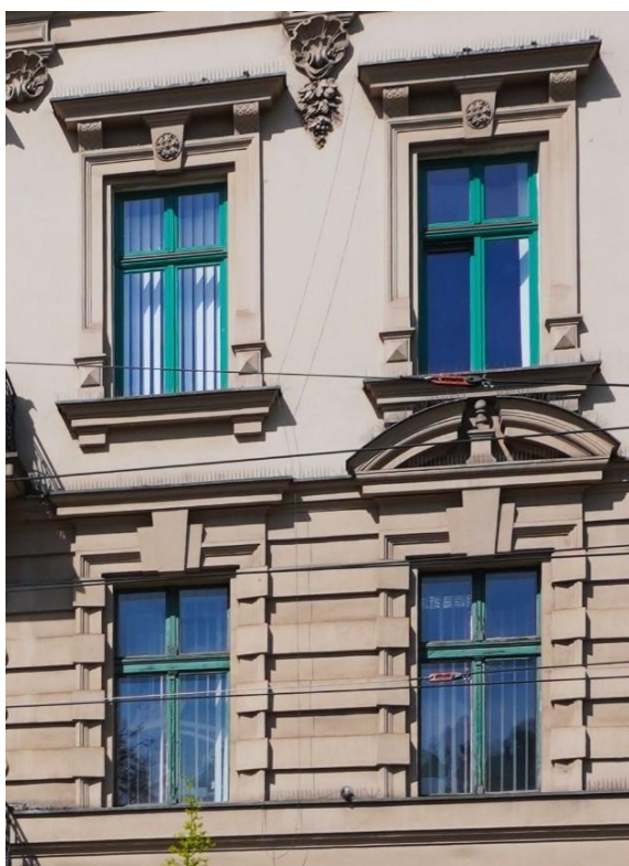
Fig. 6. Krakow, ul. Basztowa 23, an example of renovation and reconstruction of a window. Source: author.
