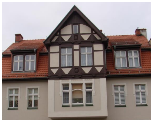
Fig. 11b. Zielona Góra. The tenement's a bay window at 18 Bolesława Chrobrego Street decorated with a half-timbered structure and carving. Source: autor's photo
