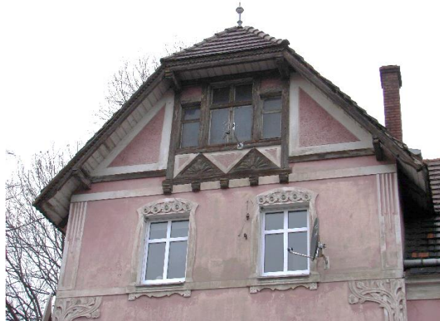
Fig. 10b. Zielona Góra. The villa a gable break at 13 Mikołaja Kopernika Street has ornaments made in the skeleton technique. Source: autor's photo
