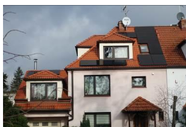
Fig. 22. Photovoltaic panels installed on the roof of the studied building. Source: Author, February 2022.
