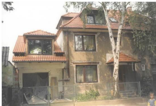
Fig. 12. The house during expansion and a major renovation in the mid-1990s. Source: Photo by the author.
