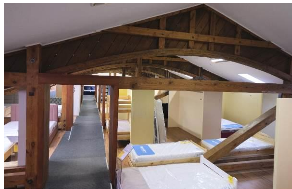
Fig. 14. The Forester's House. View of one of the girders of the roof structure above the auditorium. Photo 2024. Source: author.
