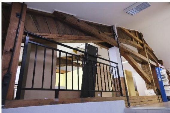
Fig. 13. The Forester's House. View of one of the girders of the roof structure above the auditorium. Photo 2024. Source: author.
