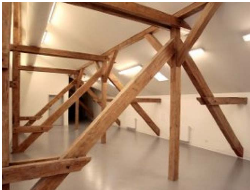
Fig. 18. The exposition of the construction of a timber roof truss in the attic, the front bay of the building, 2015. Source: photog. by M. Tuszyński
