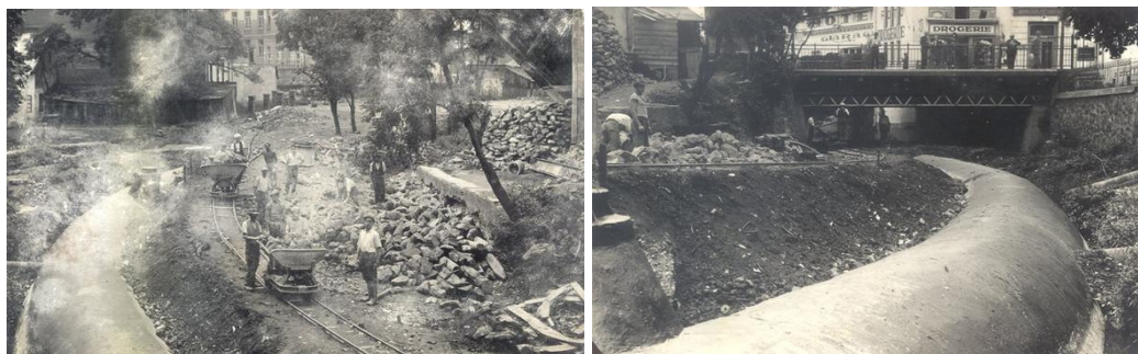
Fig. 8. The process of burial of the Small Uzh River in 1936, when Uzhhorod was part of Czechoslovakia [11]
