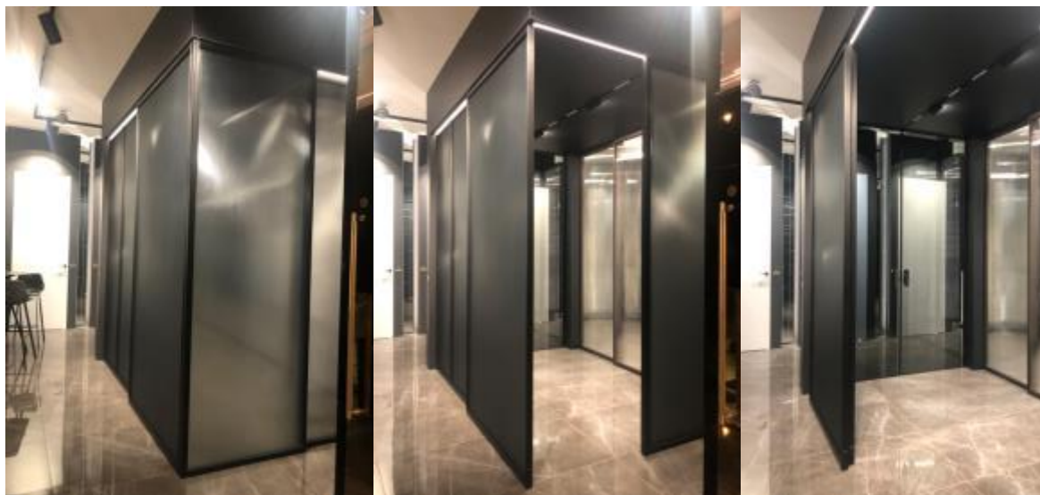
Fig. 5 Photos of the assembly of mobile wall panels for the corner and cubic system. Source: Photos from the collection of PIU Design
