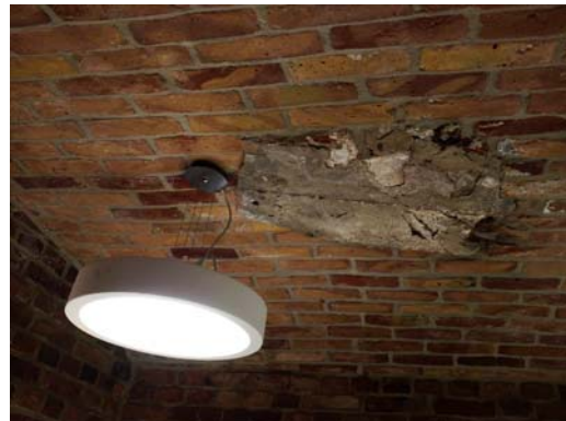
Fig. 15. "Repair" of damaged ceiling by previous owners. Source: K. Wierzbicki, October 2016
