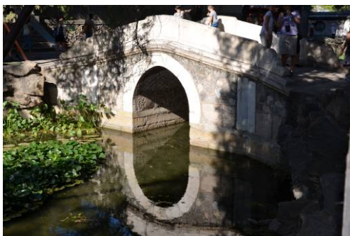
Fig. 10. Footbridge - a harmonious detail of the park around the palace. Phot. by Wojciech Kosiński
